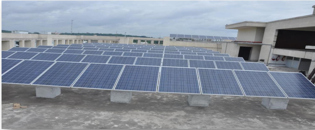
125 kW Grid Connected at Nagpur Municipal Corp, Nagpur
