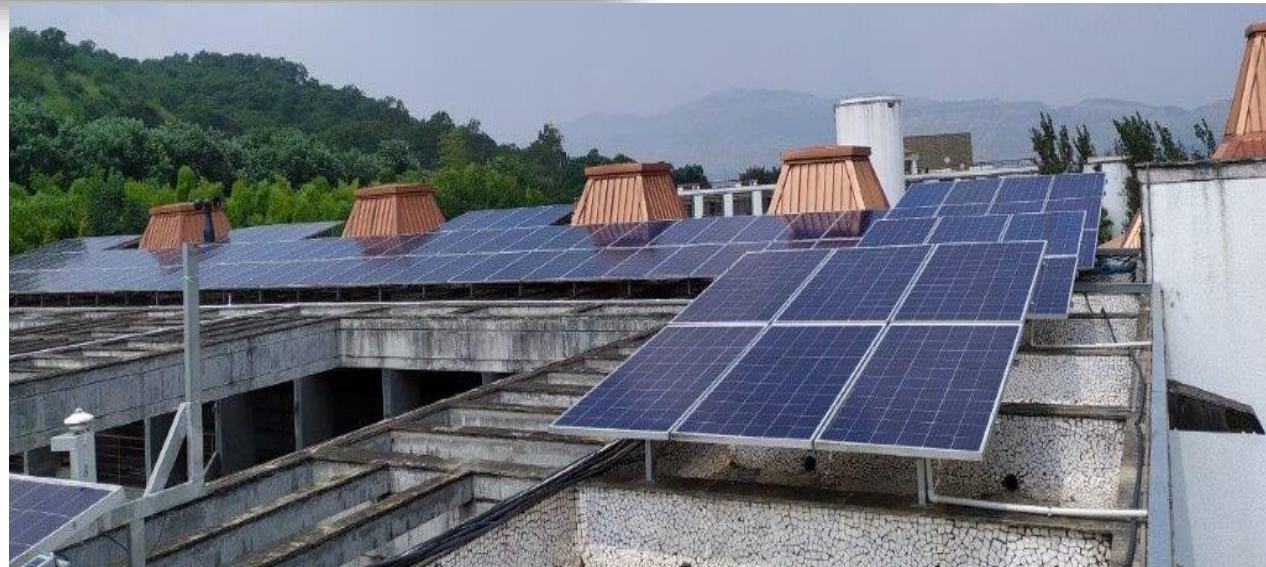
200 kW Grid Connected, KIAMS at Pune.
