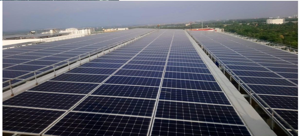
720 kW roof top solar PV system installed at SLK, Bangalore
