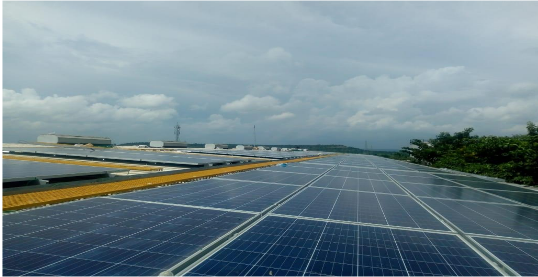
350 kW Grid Connected system on Industrial roof at Taniya Industries, Nagpur
